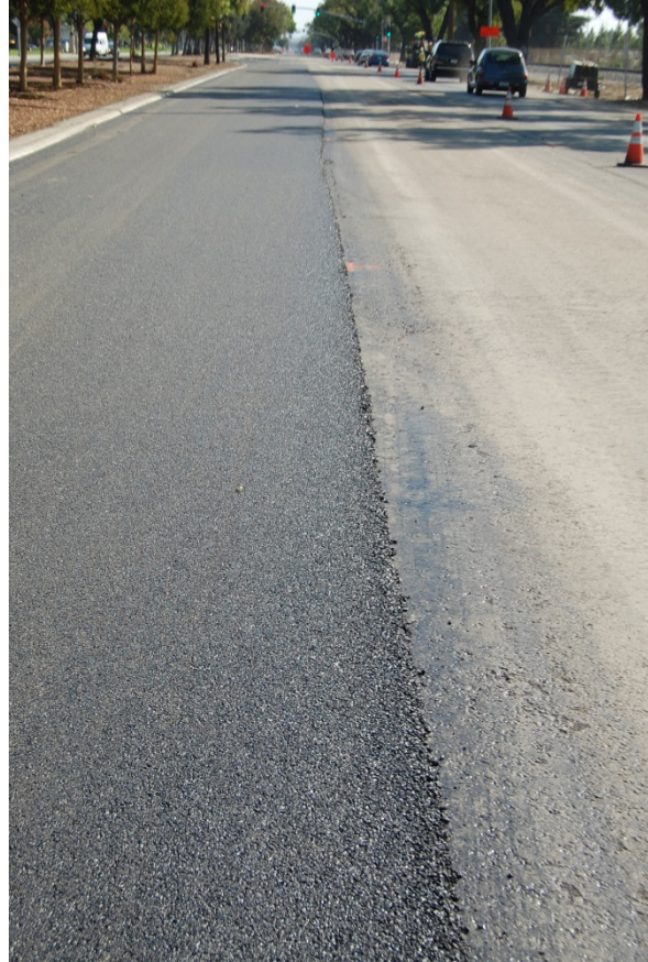
A mid-construction photo of the cold-in-place recycling process on Monterey Road in the southbound lanes. The left lane of the street has been reconstructed and repaved and is ready for traffic, but the right lanes have not yet been repaved with the surface material, which is made of asphalt with 19% recycled rubber tires. Photo by Jeralee Anderson, Greenroads Foundation.
