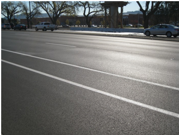
New rehabilitated pavement on Monterey Road. Photo by Patrick Hess, City of San José.
