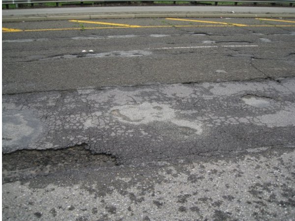
Pavement condition before reconstruction. Photo by Mike Witkovski, City of San José.
